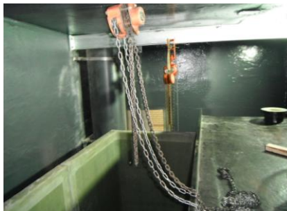
Tank Dimension: Two rectangular tanks (2.8m large x 3m long x 2.8m height) Access Dimension: 1.5m large x 2m height
