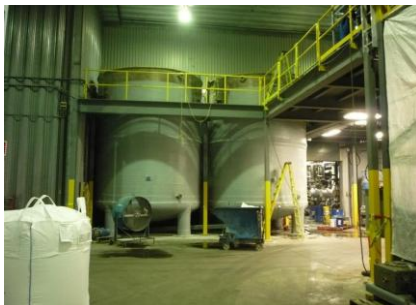
Tank Dimension: Two FRP mixing tanks (4.3m Ø x 7.6m height) installed on-site Access Dimension: 3m large x 3m height
